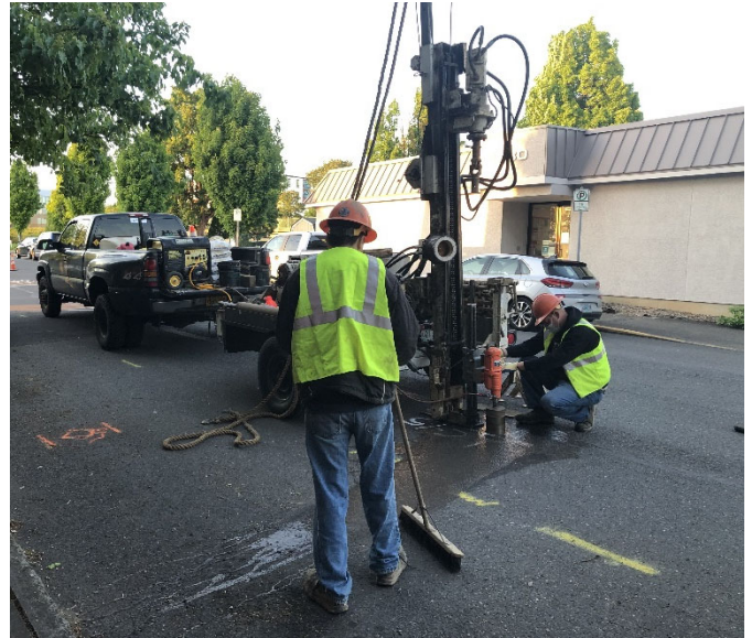
Construction team doing field work in the project area. As with field work, construction will use tools like brooms to capture and remove loose dirt and debris from construction activities, machines and vehicles during and after the work.
